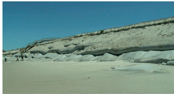
Figure 9. General aspect of some bottom geotextile layers after the high tides late in the winter of 2006, in April (Adapted from [12]).
