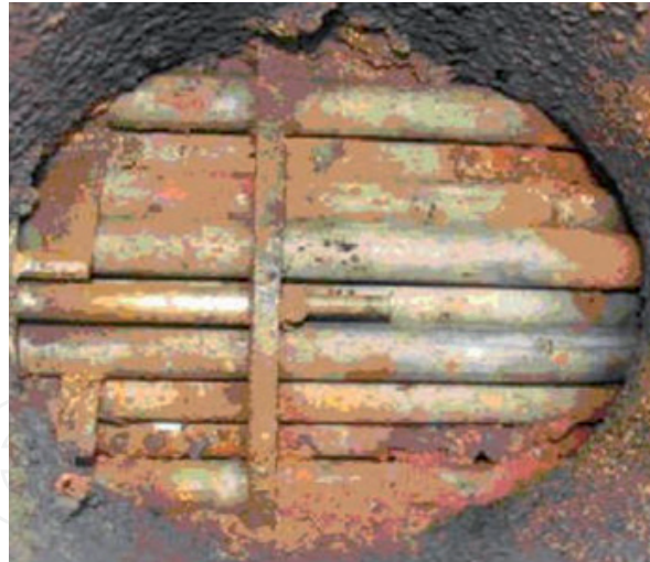
Figure 4. Oxides of corrosion in the tubes of a heat exchanger (H&C Heat Transfer Solutions Inc. 2013).
