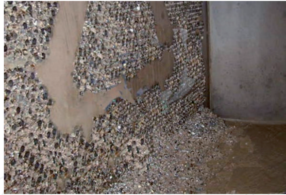
Figure 1. Presence of mussels in the water box of a condenser (Source: By courtesy of Nuclenor).
