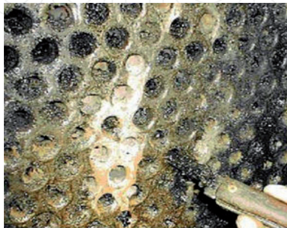
Figure 3. Residue of hydrocarbon in the tubes of a heat exchanger (Source: By courtesy of H&C Heat Transfer Solutions Inc. 2013).
