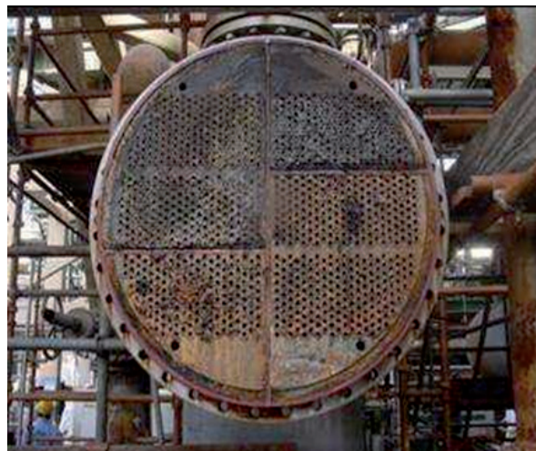
Figure 2. Tubular heat exchanger in maintenance due to the presence of biofouling in its tubular bundle (Source: By courtesy of Merus-the water conditioner company).
