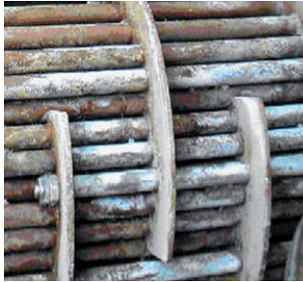
Figure 6. Precipitated salts in the tubes of a heat exchanger (Source: By courtesy of H&C Heat Transfer Solutions Inc).
