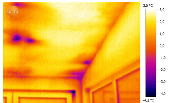
Figure 3.6 Thermal bridges on the ceiling
