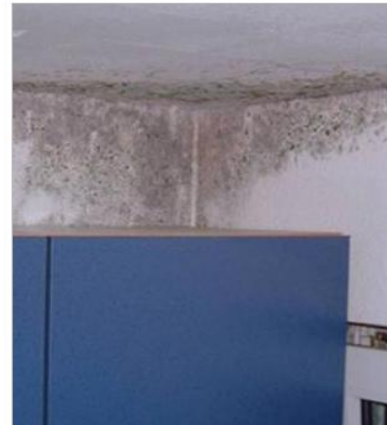
Figure 4.67 Fungus in the corner of the wall, which is the result of too high air humidity
