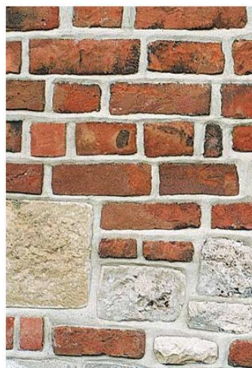
Figure 4.23 Mortar with additive of trass prevent efflorescence of lime.
