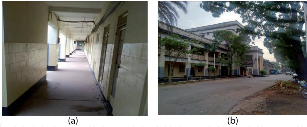
Figure 6. (a) Corridor along the Ministry of Water Resources and (b) Ministries of Justice at the background and Water Resources at the foreground in need of renovation.
