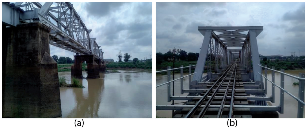
Figure 10. (a) Railway line bridge across river Kaduna and (b) intricate steel works carrying the rail line across river Kaduna.
