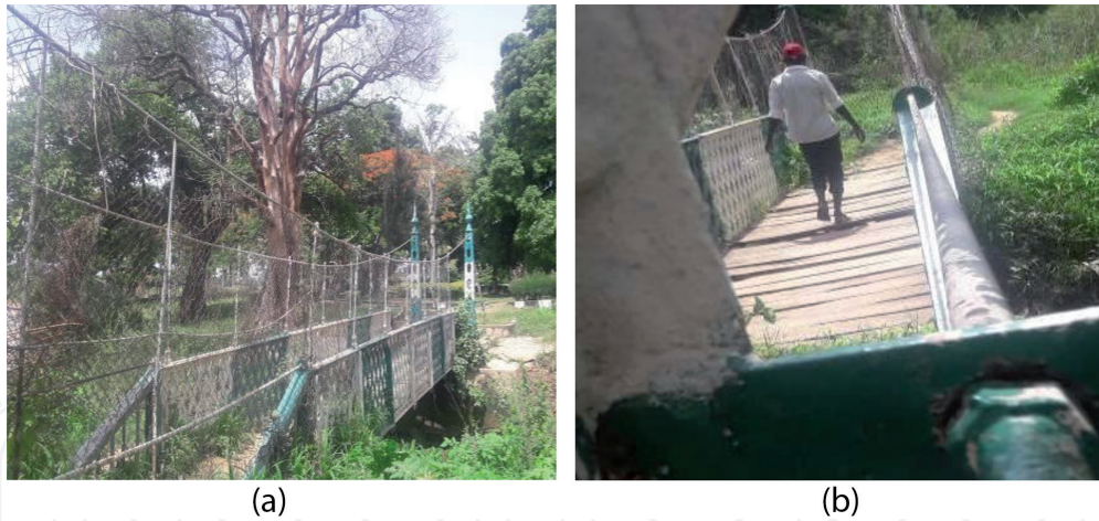
Figure 9. (a) Lord Lugard Bridge at Gamji Gate showing the steel frame across one of the streams to river Kaduna and (b) bridge showing the timber planks serving for foot passage.
