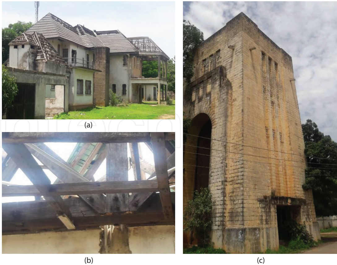
Figure 4. (a and b) Lord Frederick Lugard residence as you approach and the roof trusses showing well-seasoned timber bolted and secured for about a century. (c) Lord Frederick Lugard residence Water Tower often used as a watch tower during early days of Kaduna township development.
