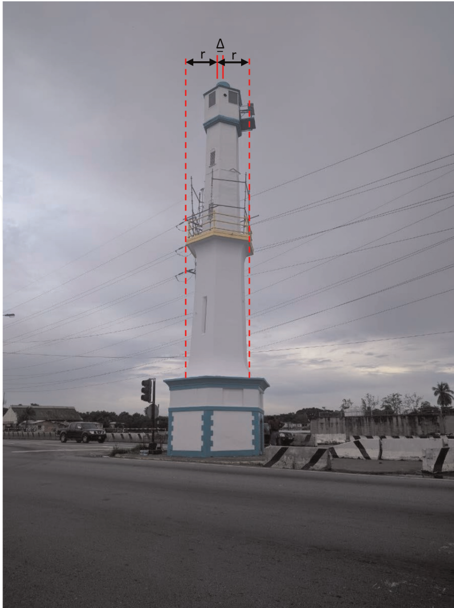
Figure 14. Leaning lighthouse tower at the Port Area. See the displacement \Delta at the top of the structure due to the soil subsidence at its foundation.
