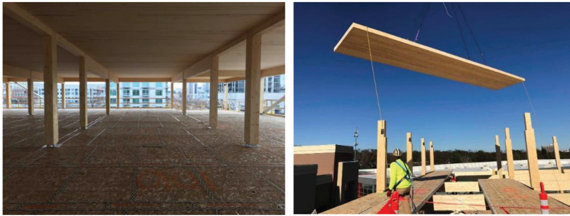
Figure 15. Seven-story T3 Atlanta building comprising DLT floor and roof panels in USA (Source: Photos obtained from StructureCraft [18]).
