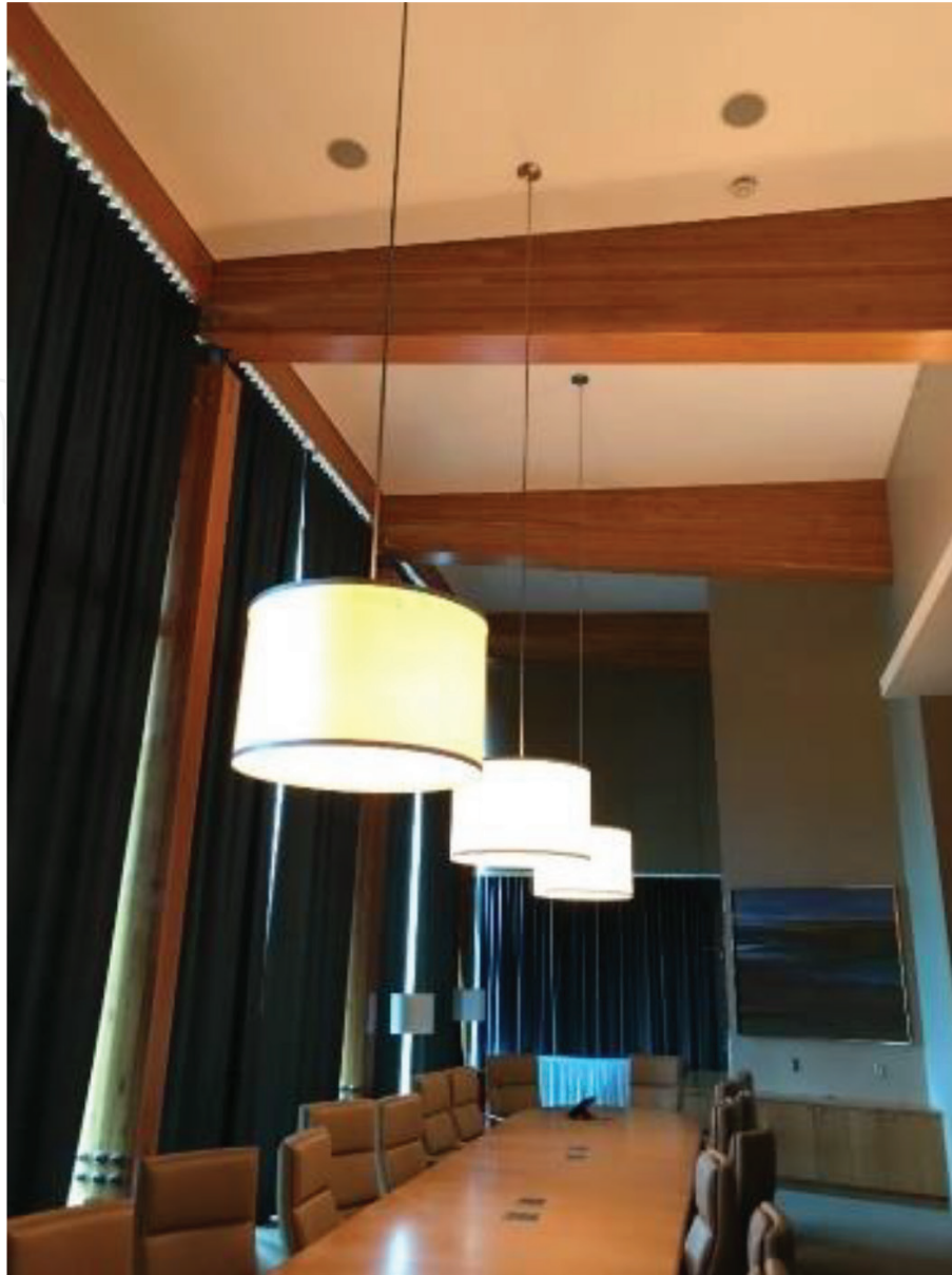
Figure 6. Conference room built with GLT beams and columns at the University of New Brunswick, Fredericton, Canada.
