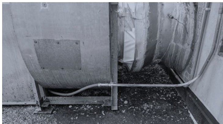
Figure 3. Pigeon nests under a HVAC machine on top of the Biology building on TTU campus.
