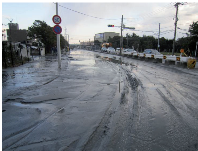
Figure 8. Liquefaction damage in Chiba Prefecture at East Japan (after Funabashi city data in Chiba Prefecture).
