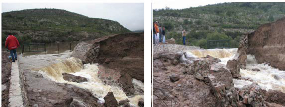
Figure 4. Overflow and failure of the spillway of the La Salitrera dam, in 2010.
