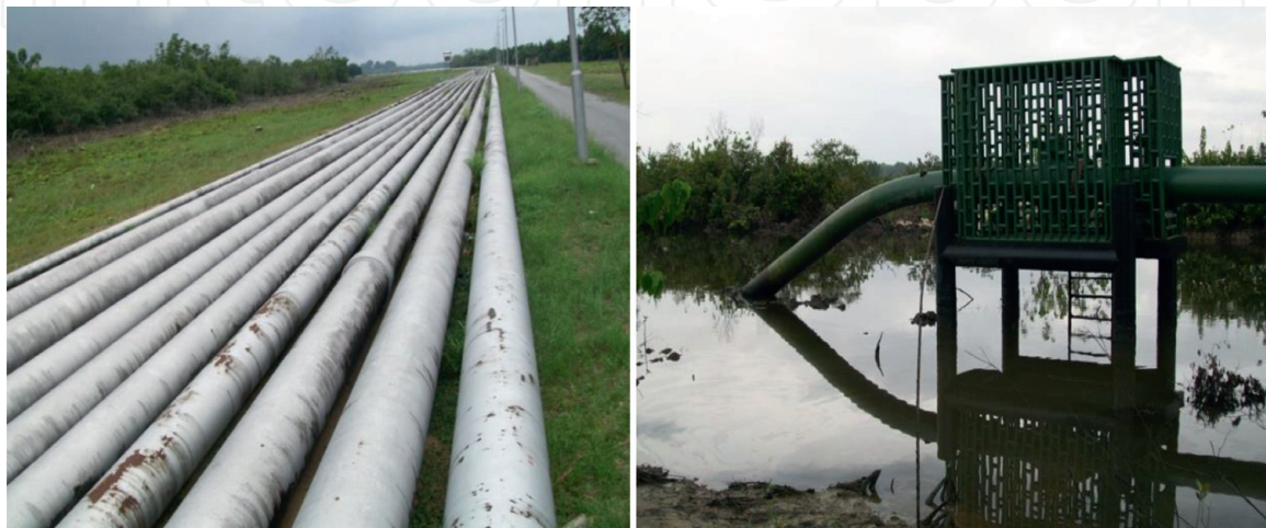
Figure 5. Crude oil pipeline and well head situated in reclaimed coastal area in the Niger Delta, Nigeria.
