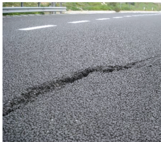
Figure 12. Detail of a fracture in the asphalt at the beginning of the landslide phenomena.
