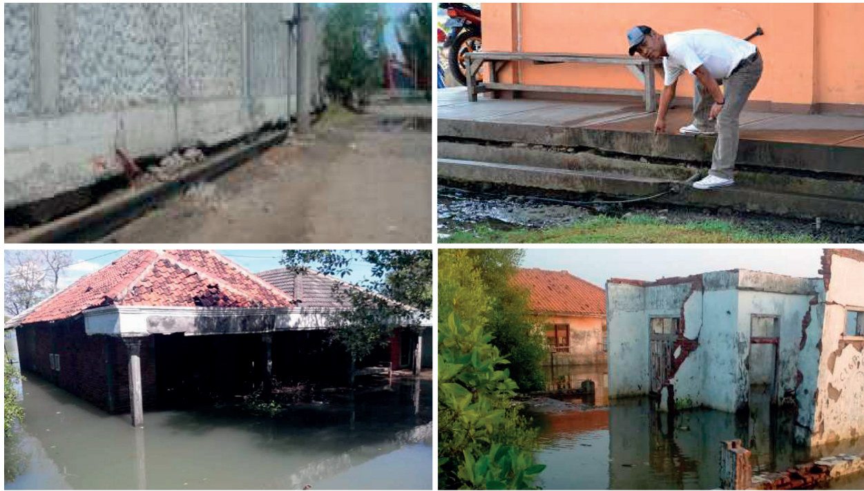
Figure 7. Pictures of the impact of subsidence (e.g. cracks in buildings and infrastructures and tidal inundation) in other regions of Indonesia (source: authors).
