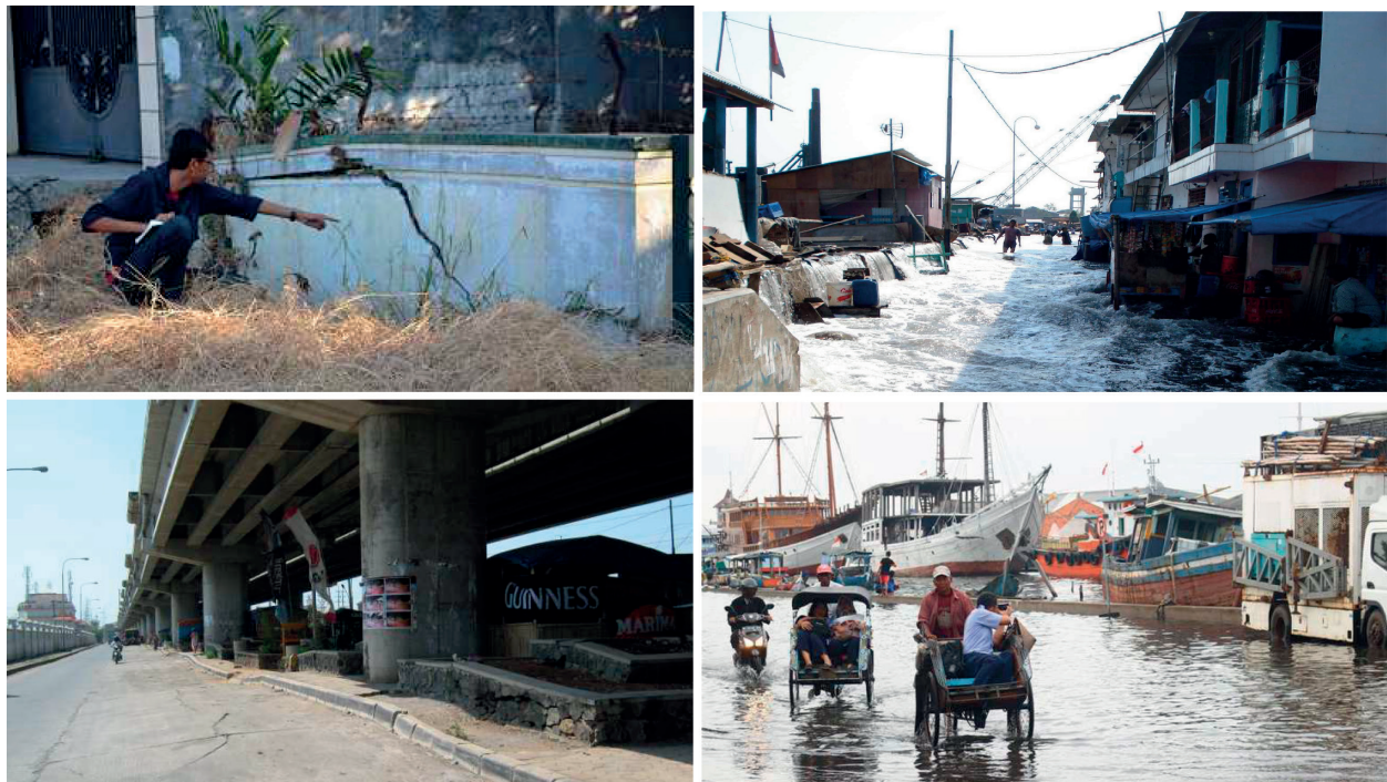
Figure 6. Pictures of the impact of subsidence (e.g. cracks in buildings and infrastructures and tidal inundation) in Jakarta, Bandung, and Semarang (source: authors).
