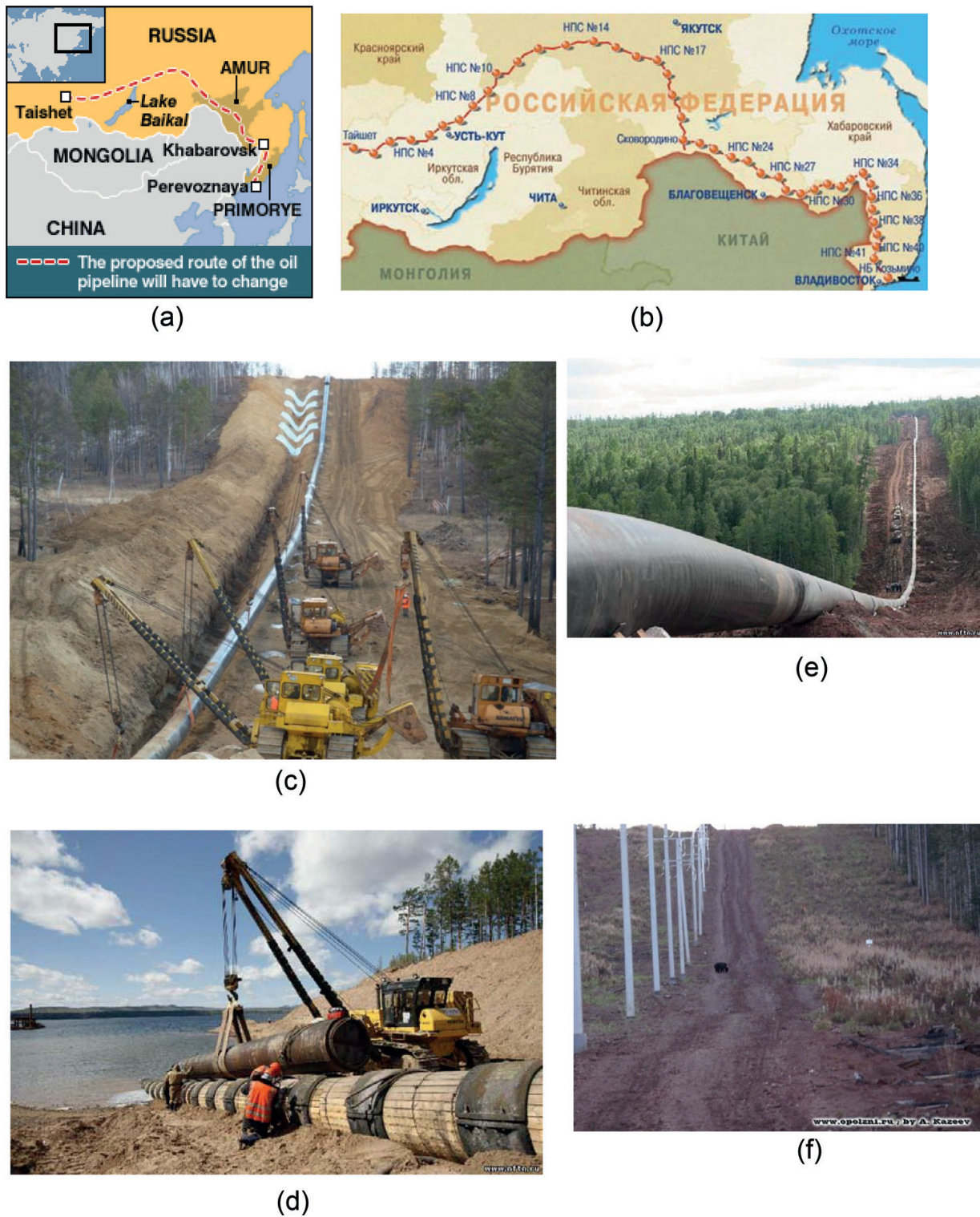
Figure 8. (a, b) Eastern Siberia-Pacific ocean oil pipeline (c, d, e, f). ESPOOP construction.
