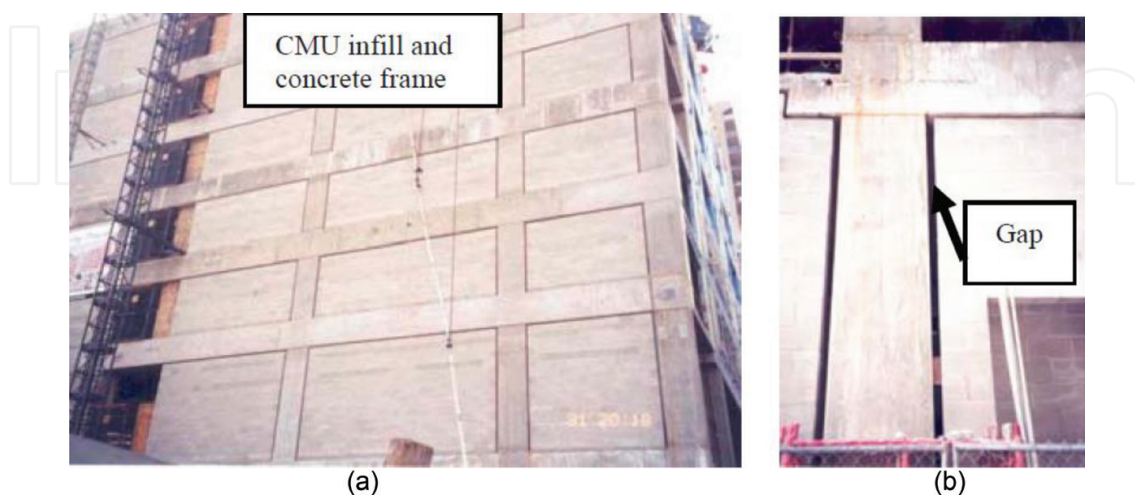
Figure 4. Use of large gaps between infill backup wall and frame in a Seattle building: (a) view of several stories of the building and (b) close-up view of gaps between column and infill walls [Photo by Ali M. Memari].
