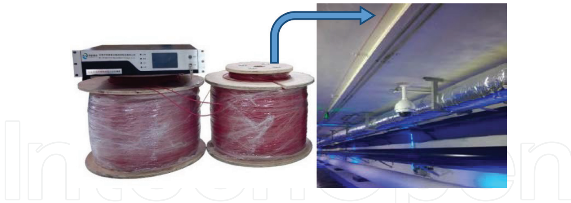
Figure 10. Application of the DTS system to fire monitoring in urban underground comprehensive pipe corridor.
