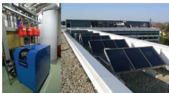
The Fraunhofer ISE institute building and SorTech adsorption chiller in the technical room (sources: Fraunhofer ISE) [34]
