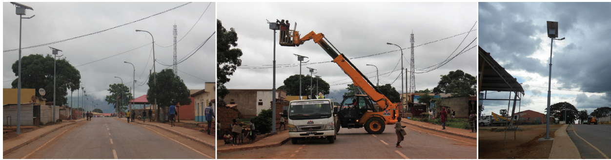
Figure 9. Solar autonomous public streetlight installation in Cuimba, Angola, 2017.
