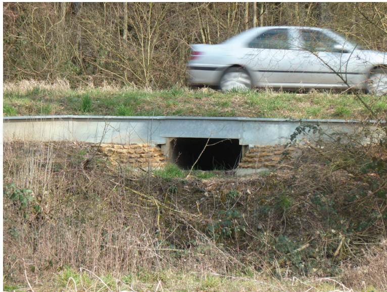
Figure 3. Ecopassage designed for the migration of amphibians along the road RD657 in NE France. This ecopassage allowed the migration of amphibians such as the common frog Rana temporaria and the common toad Bufo bufo . A concrete tunnel, with the floor covered by the soil, allows the animal crossing. A metallic barrier prevents the animals to access the road and directs them toward the tunnel entrance. This ecopassage is located below the local road joining Novéant-sur-Moselle to Arry in Northeastern France (photograph by Alain Morand, CEREMA-EST).
