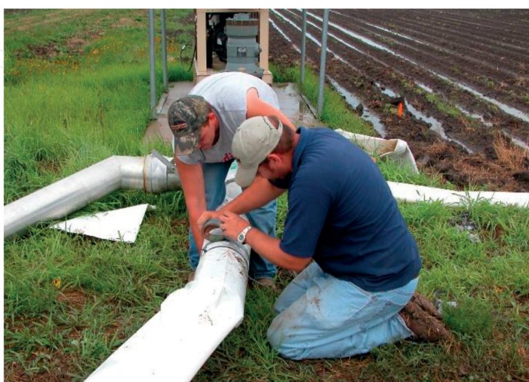
Figure 2. Connecting plastic tubing to well pipe with zip ties and duct tape.
