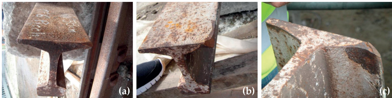
Figure 16. Track reference stake no. 24 photographed after its extraction from the track ballast. (a) In the foreground: flange of the track reference stake with damaged edge; in the background: view of the concrete plinth; and (b) and (c) details of the damaged edge.
