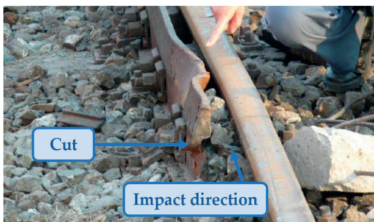
Figure 19. Check rail opposite to the wing rail photographed during the investigations on the accident site conditions.
