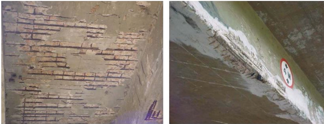
Figure 4. Corrosion on the reinforced concrete of a viaduct [41].
