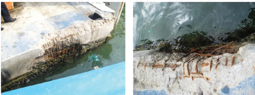
Figure 6. Corrosion of reinforced concrete in Qeshm port, Iran [45].
