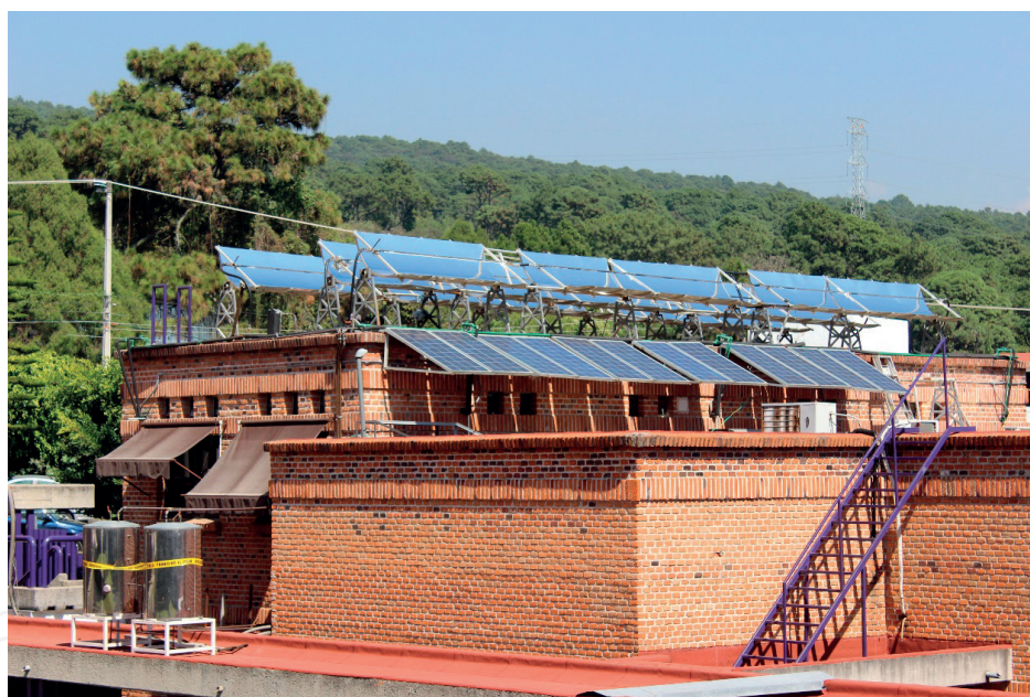
Figure 2. Photograph of the thermal and photovoltaic solar systems on the building roof.
