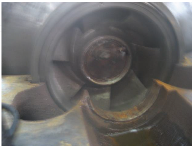
Figure 2. Failure scenario of the centrifugal pump showing the fractured rotor shaft.
