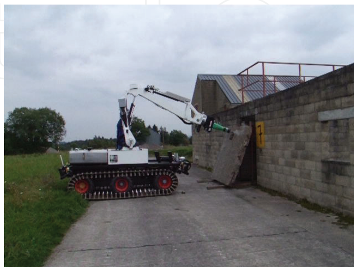
Figure 16. The LUGV uses its jackhammer to breach through a concrete plate (Source: ICARUS).
