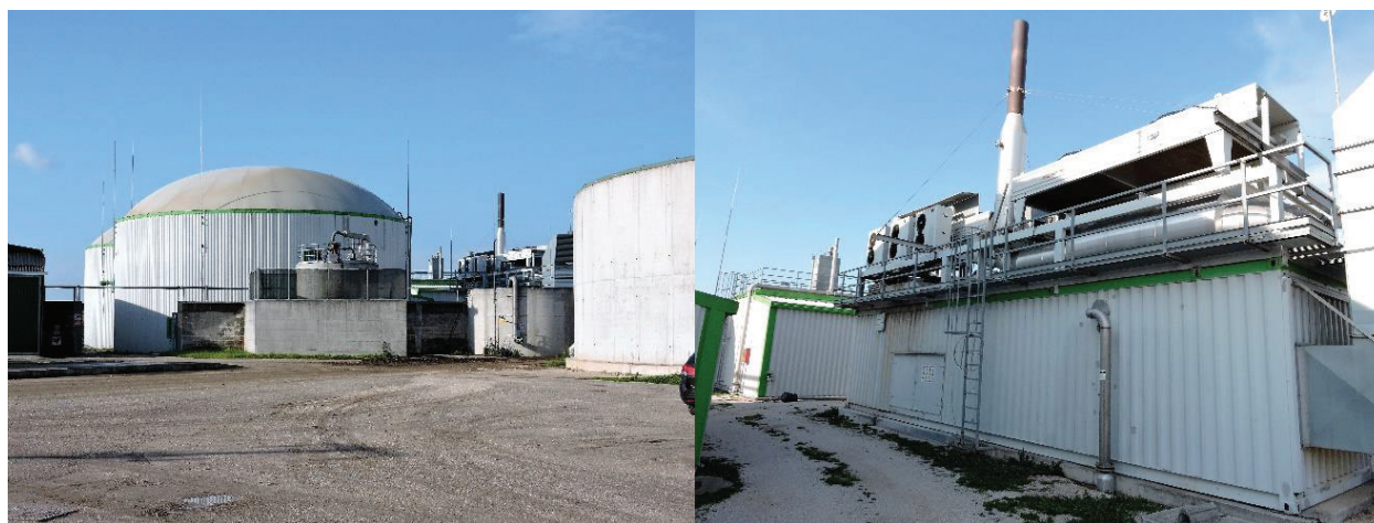
Figure 3. Power generation plant (1 Mw) fed with wet olive husks and wastewaters from the olive oil extraction. Biogas is generated in the digester (right) and stored (left), then converted into electricity. Installation Friel Ionica Srl - BTM Srl spinoff of the University of Pisa, located in Manduria (Taranto, Italy) (Source: Marco Nuti).
