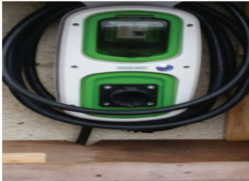
Figure 14. Domestic electrical vehicle charger.
