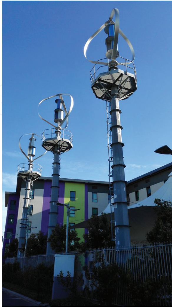
Figure 4. Huebner-Giessen 3 kW wind turbines.
