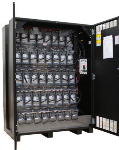
Figure 7. The batteries used to store generated energy.
