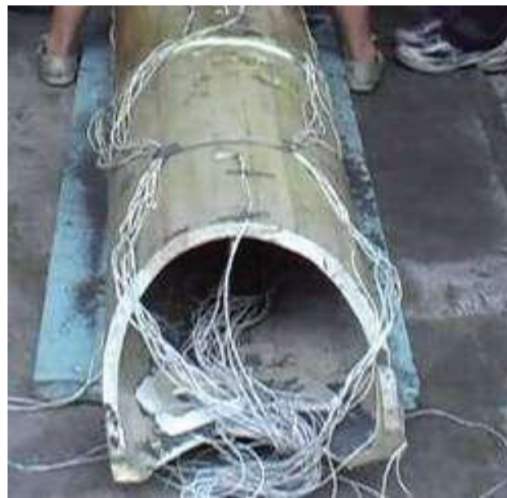
Figure 14. The fracture of the liner with soft isolation layer (right tunnel) in case 2.
