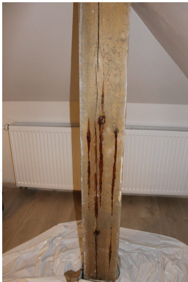
Figure 10. Resin melting in pine wood after exposure to microwaves radiated in practice by the 0.6 kW SAURUS device made in Italy (photo by CARSEKT).
