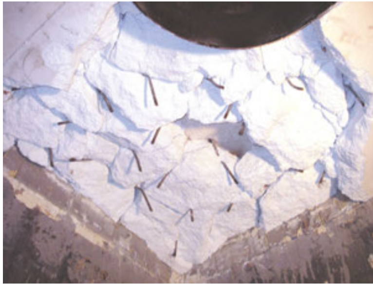
Figure 12. The part of the combustion zone structure in the heating unit used in oil refineries damaged by explosive spalling (metal anchors can be seen on the photograph) [29].
