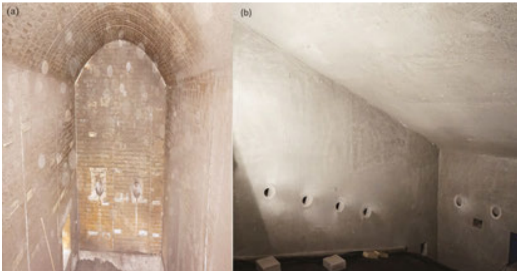
Figure 2. Biofuel boiler lining made of (a) fired bricks and (b) castables.
