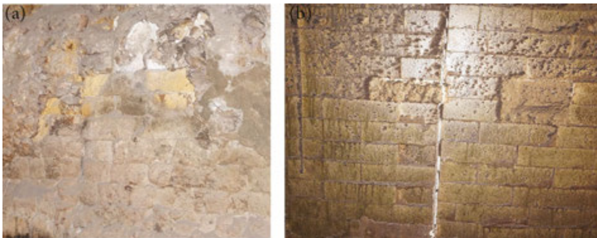
Figure 15. View of lining made of not alkali resistance fire clay bricks after 6 months of boiler operation (a) and made of alkali resistance fire clay bricks after 8 months of boiler operation (b).
