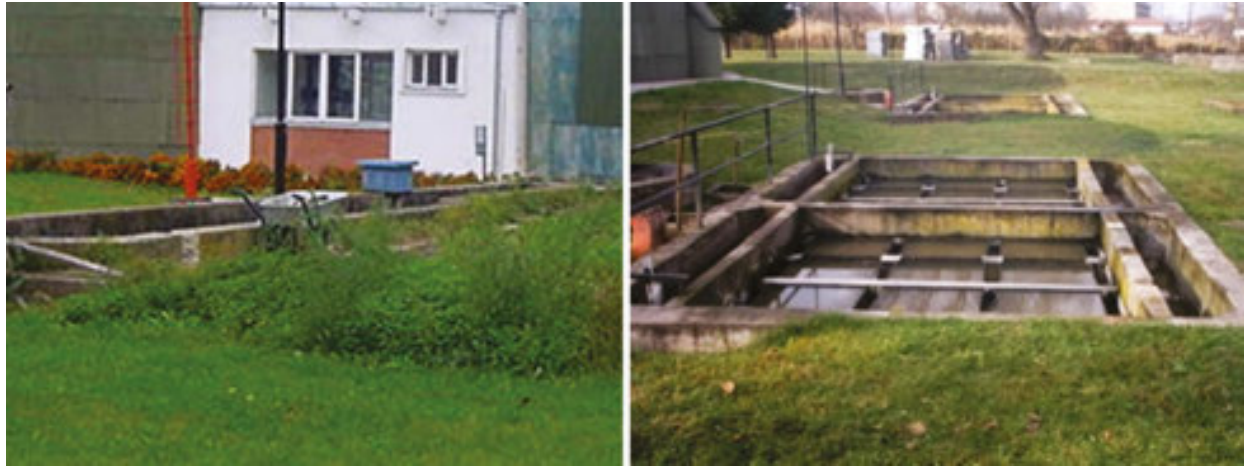
Figure 6. Inlet structure and efficient settlement tank on the WWTP Sokobanja.
