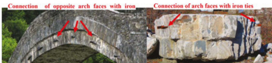
Figure 12. Iron ties used to connect the two opposite faces of the primary arch in Plaka Bridge.
