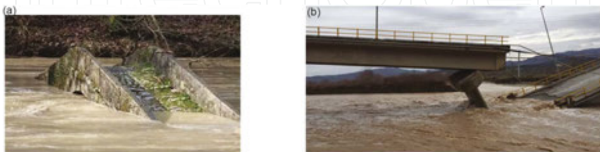
Figure 49. (a) Almost total flooding of a stone masonry bridge and (b) tilting of a mid-pier and partial collapse of the Diava-Kalampaka reinforced concrete bridge in Thessaly, Greece (16th January, 2016).
