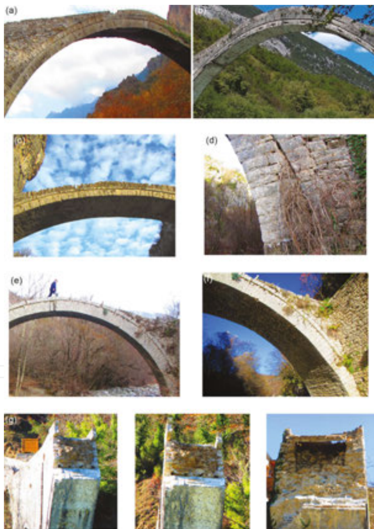
Figure 10. (a) Konitsa Bridge with the primary and secondary arches of the central span; (b) Plaka Bridge with the primary and secondary arches of the central span; (c) and (d) Kokorou Bridge with the primary and secondary arches of the central span; (e) and (f) Kontodimou Bridge with the primary and secondary arches of the central span; and (g) stone-masonry construction visible for the internal part of the mandrel walls of the remaining parts of Plaka Bridge.
