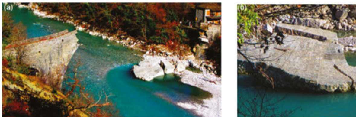
Figure 50. (a) View of the Plaka Bridge after the collapse from the West bank. Note the total destruction of the mid-pier (see also Figure 7d ). (b) Close-up of the total destruction of the mid-pier of Plaka Bridge (see also Figure 7d ).
