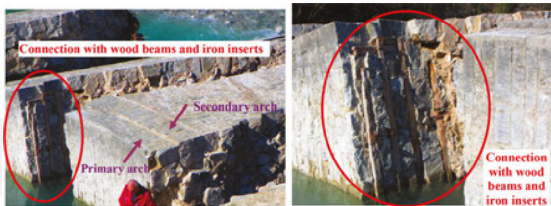
Figure 11. Connection with wooden beams and iron inserts between the primary and secondary arches of the Plaka Bridge.
