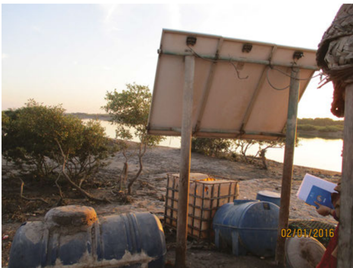
Figure 9. Broken solar panels require maintenance and repairs; the only source of power to recharge torch and mobile phone batteries.
