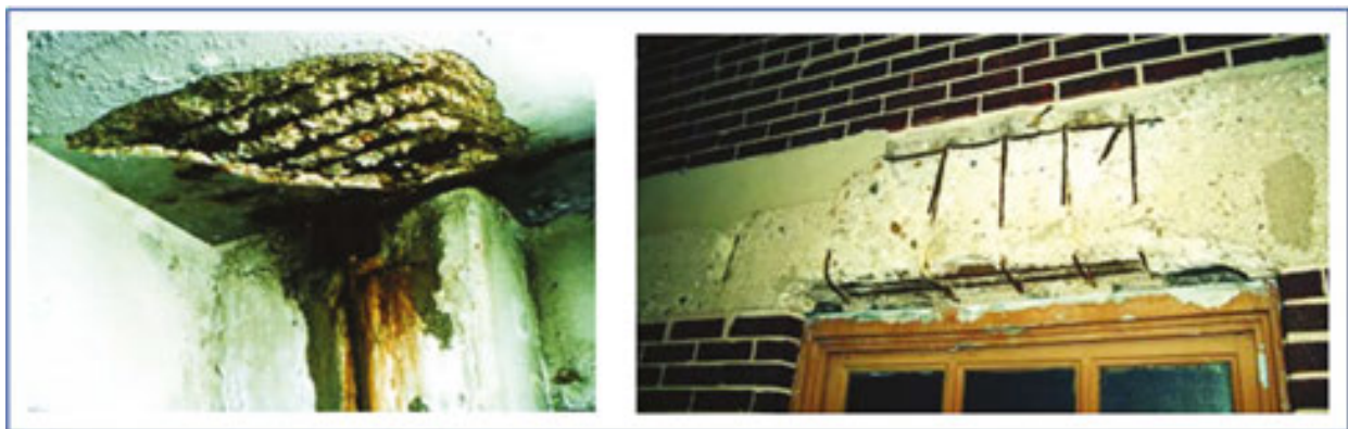
Figure 2. Deterioration of normal concrete [7].
