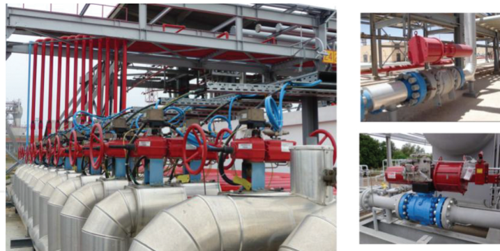
Figure 7. Example of emergency shutdown valve.
