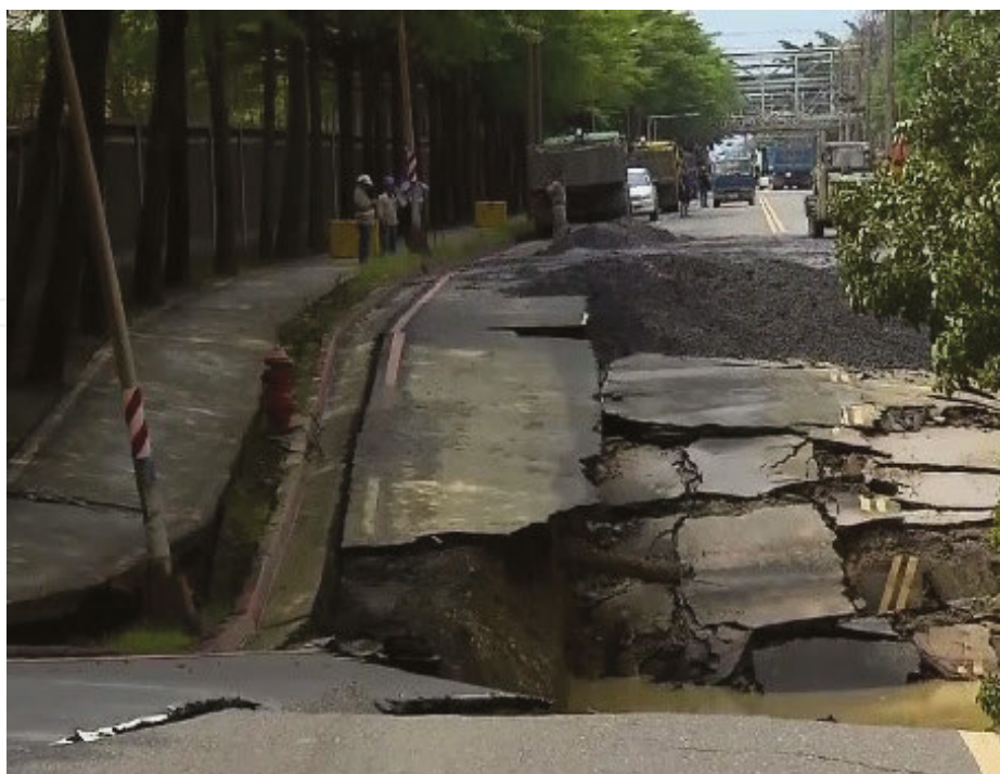
Figure 2. Destruction of roadway.
