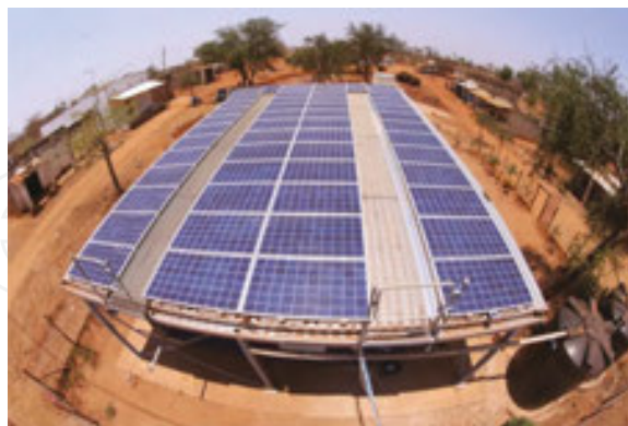
Figure 1. Makueni County 13.5 kW PV system, Kenya, Kitonyoni village market. (Phys. Org, 2013).
