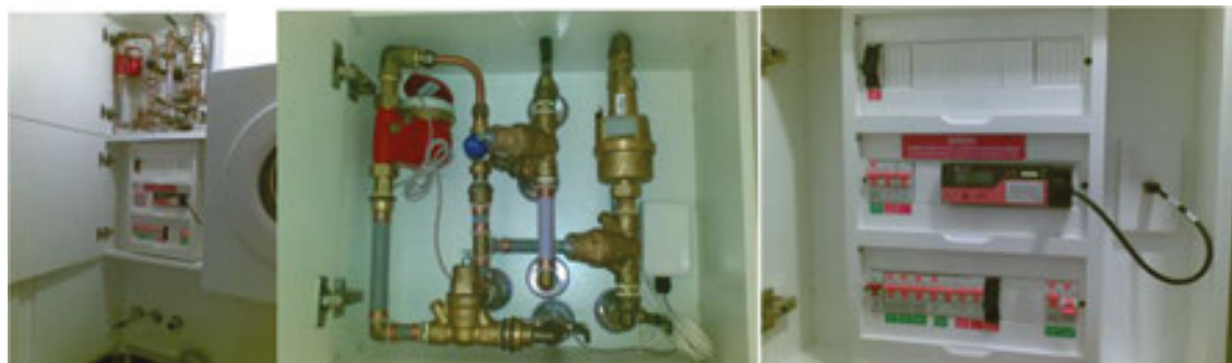
Figure 9. Meters installed at Central Park: (a) typical complete installation of meters for gas, electricity, hot water, cold water, (b) close up view of the gas and water meters, (c) showing electricity meter EM133AR installed in residential DB with Ethernet output to building IP backbone.
