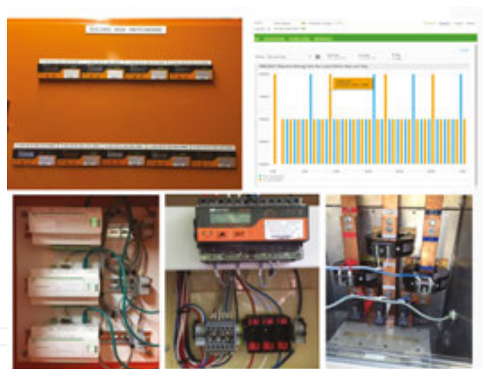
Figure 7. Installed Embedded Network Installations in 2015 at Murdoch University: from top left and left to right each row (a) 9× SATEC EM133 meters installed on main distribution board in one building, (b) chart showing output from the Schneider Electric COM510 energy server webpage, (c) showing the 3× energy servers with ethernet and modbus connections, (d) and (e) showing the EM133 smart meter installation using IPD CTs, test links and voltage fuses.
