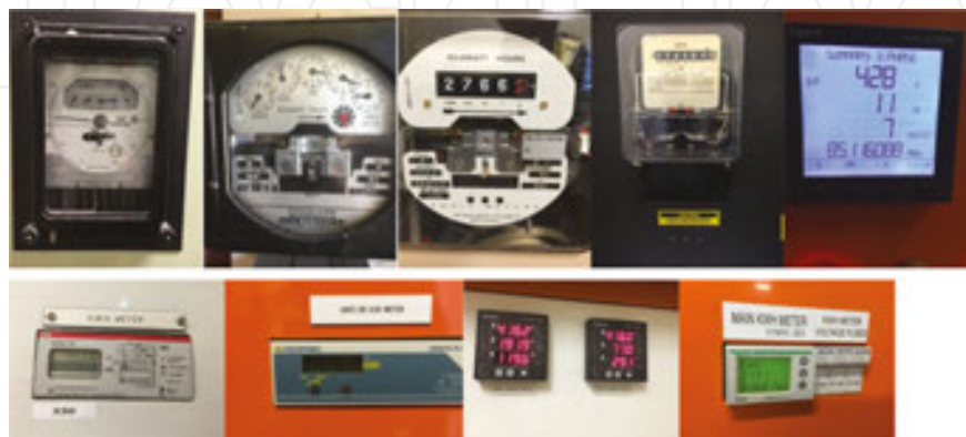
Figure 6. The variety of existing meters installed at Murdoch University.
