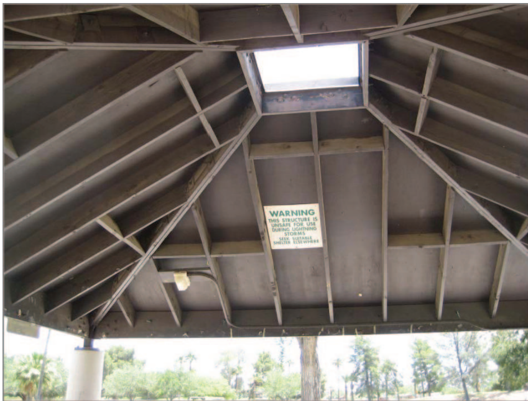
Figure 13. Lightning-unsafe small structure. Note sign recommending a safe place elsewhere rather than staying at this location (©R. Holle).
