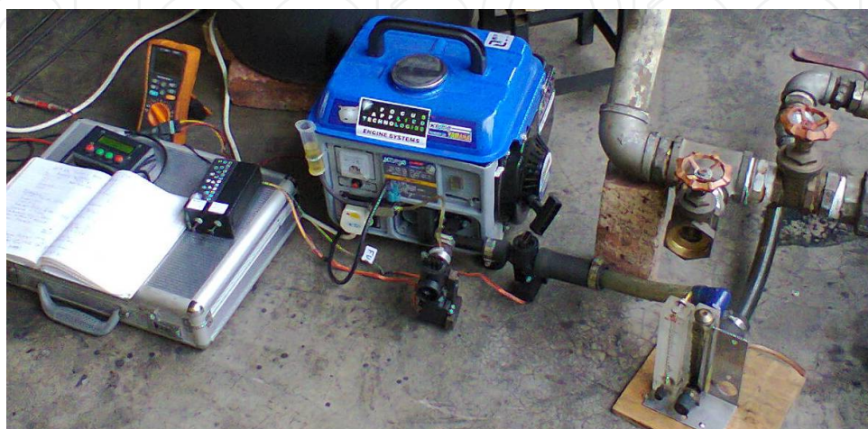
Figure 11. AFR and throttle controller are to the left of the engine, as is the digital display. Note that the gas supply system has relatively large pipes to supply the unpressurized syngas.
