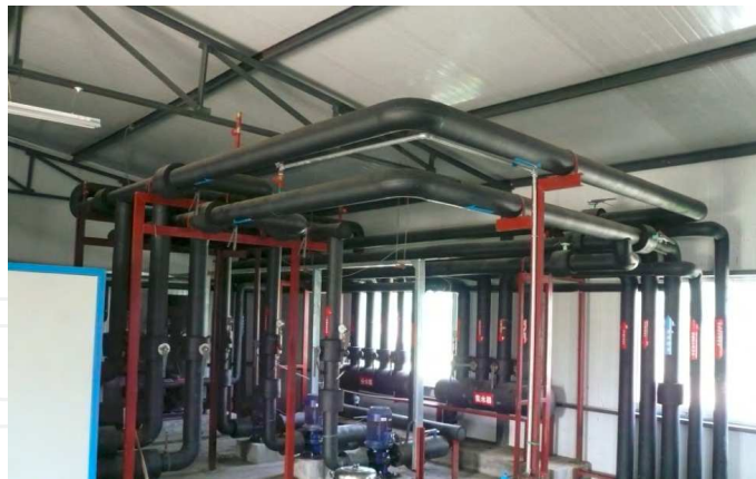
(a) The heat pump and water circulating system
