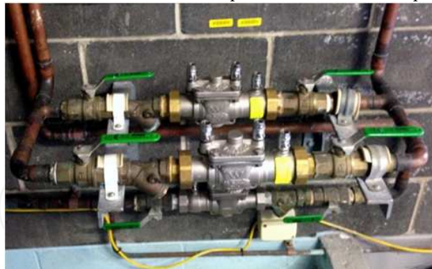
(B) A backflow device.
