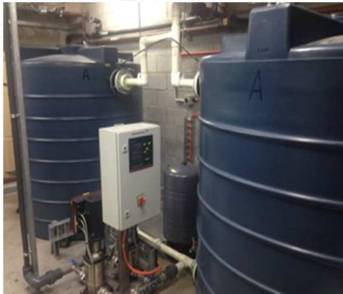
A) Two 3000L holding tanks to provide an uninterrupted water supply in case of emergency. Note also the booster pumps in the centre. These ensure an inlet pressure of at least 550Kpa
