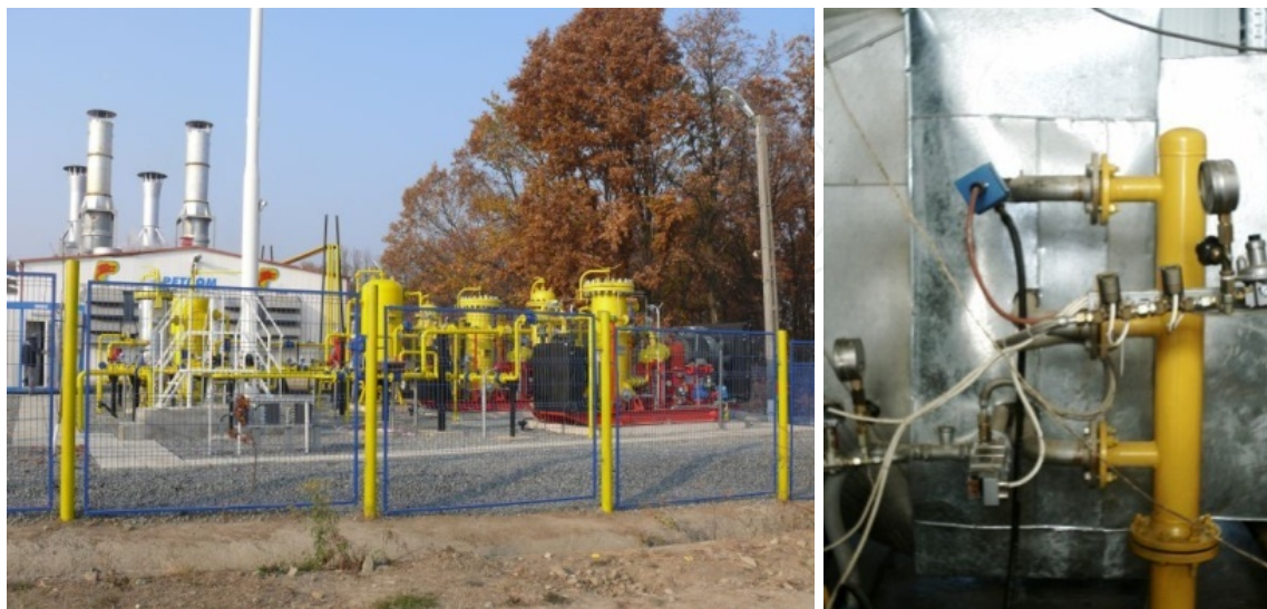
Figure 2. Cogenerative plant 2xST 18 – Suplacu de Barcau (left) and afterburning installation (right) [14, 15]
