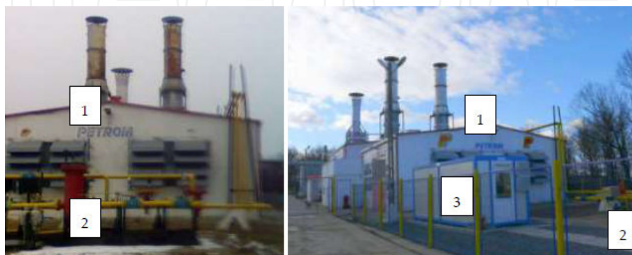
Figure 4. Control – measurement station for natural gas at 2xST 18 – Suplacu de Barcău plant (left) with booster (right) 1 – cogeneration power plant; 2 – control – measurement station; 3 – booster
