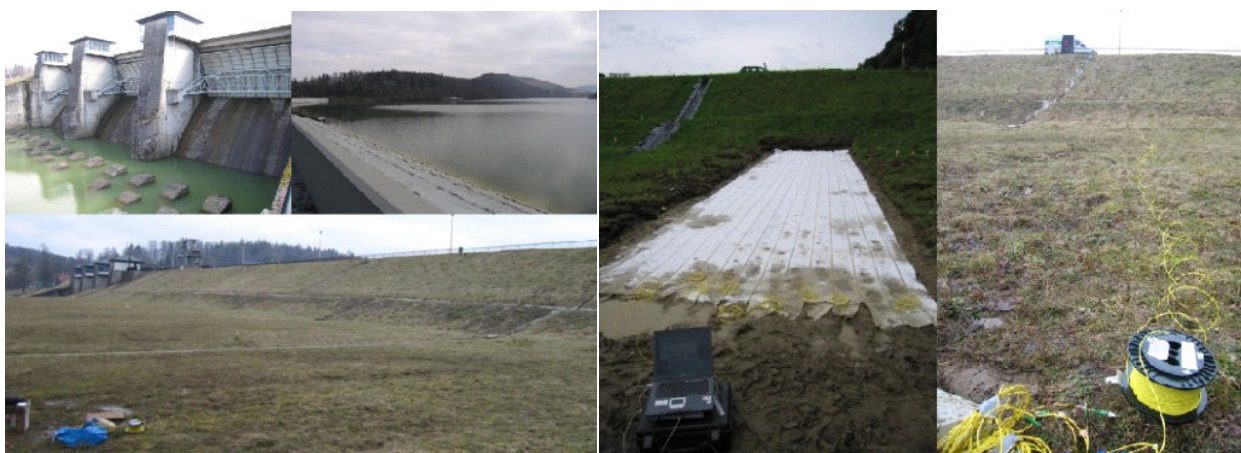
Figure 6. Gravity dam in Solina, Poland (left) and the construction site with the sensor-based non-woven geotextile before embedding in the soil and 3 years later (right).
