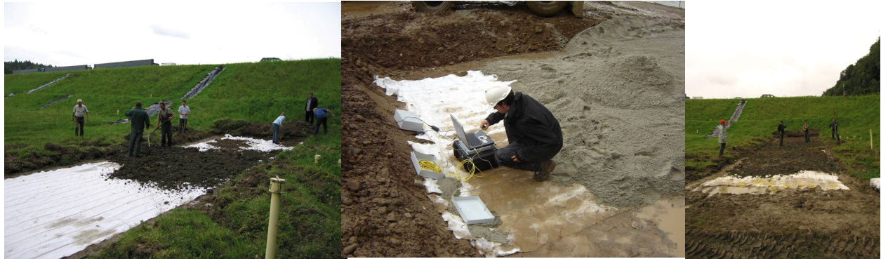
Figure 3. Installation of a non-woven geotextile containing single-mode silica fibers as Brillouin sensors in a gravity dam in Solina, Poland.
