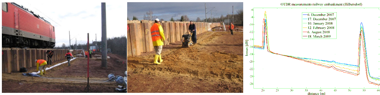
Figure 12. Installation of POF-equipped geotextiles in a railway embankment near Chemnitz, Germany (left and middle) and OTDR traces measured on the textile-integrated POF (right).
