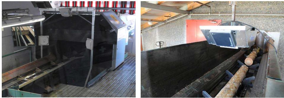
Figure 10. RFID readers in the log sorting and sawing in a saw mill.
