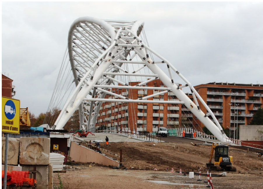
Figure 2. The Garbatella bridge seen from its western side. AE monitoring was carried out at the base of the single eastern "leg" here shown in the background.
