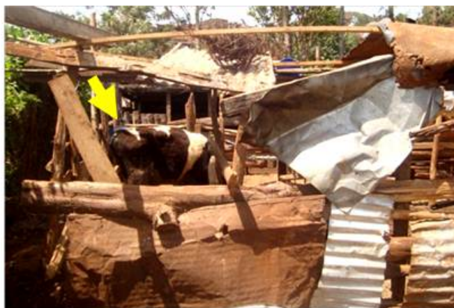
Figure 11. Collapsed iron sheet roof and sides in one of the zero-grazing units evaluated. Both the roof and side timber are broken and collapsing. Yet cows are still housed inside (arrow).
