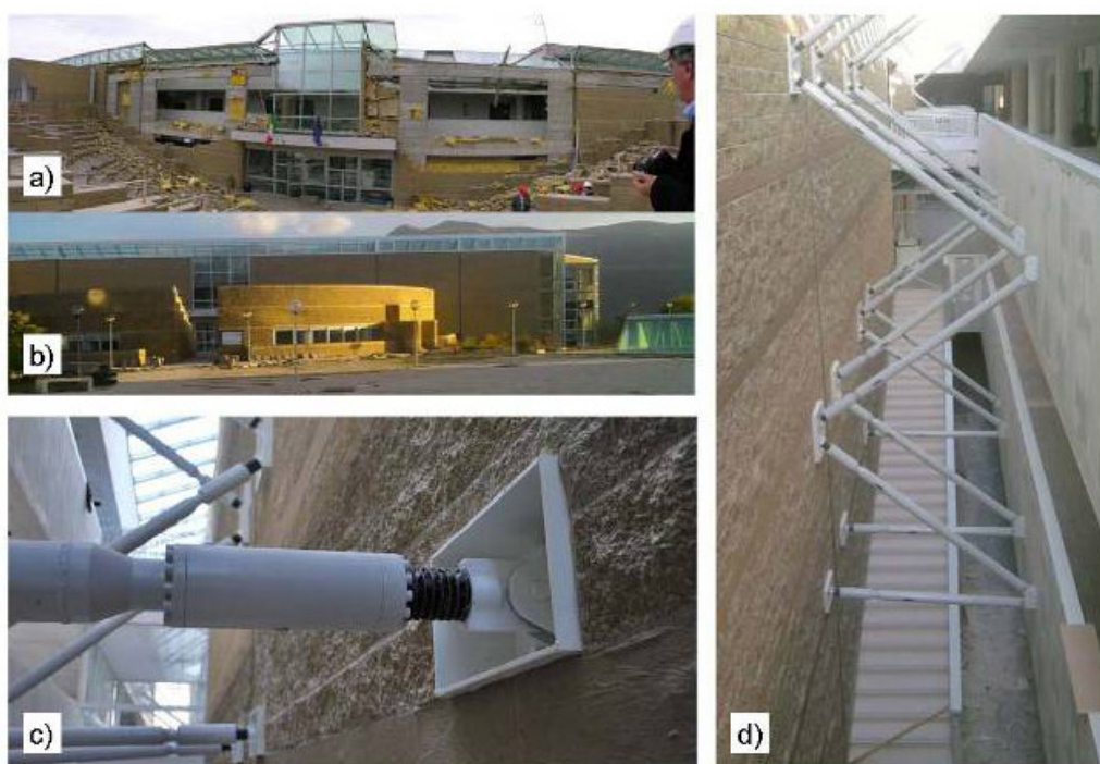
Figure 9. Reconstruction at Edifice A: a) damage scenario involving the facade, b) reconstruction of the facade, c) close view of the installed device, d) dissipative truss structures.
