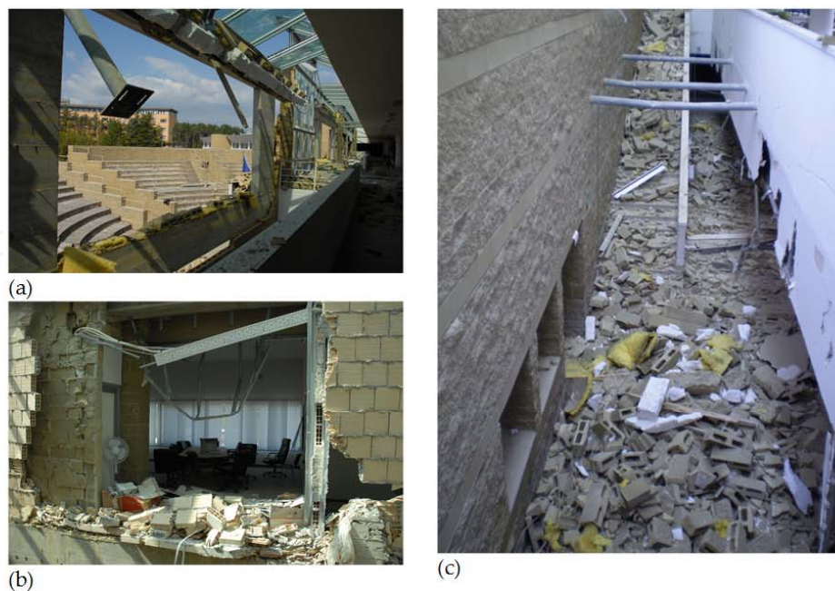
Figure 3. Damages caused by 2009 earthquake to the Edifice A: a) internal view of the main facade, b) internal partitioning walls c) heavy bricks fallen down inside the building from the facade.
