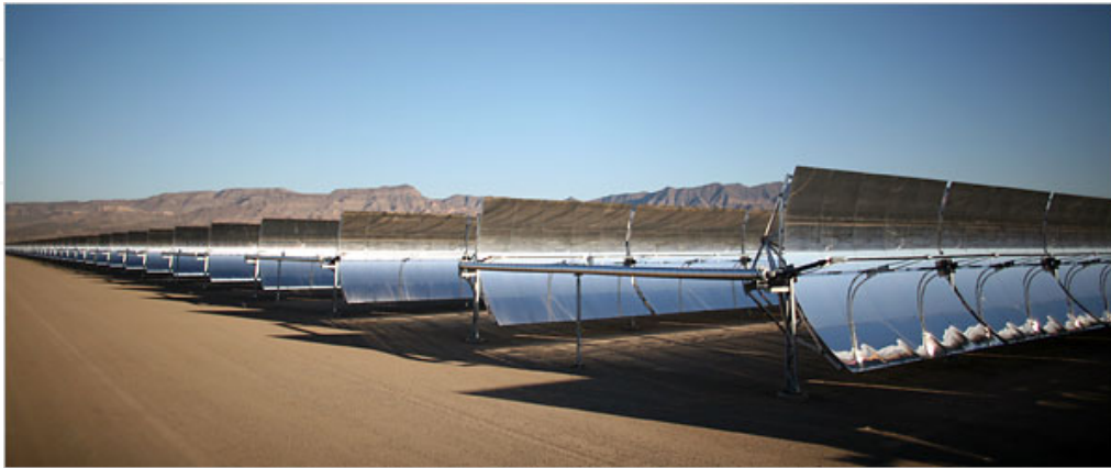
Figure 5. Parabolic-trough collectors in Nevada Solar One power plant [41].
